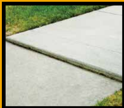
SIDEWALK TRIP HAZARD
